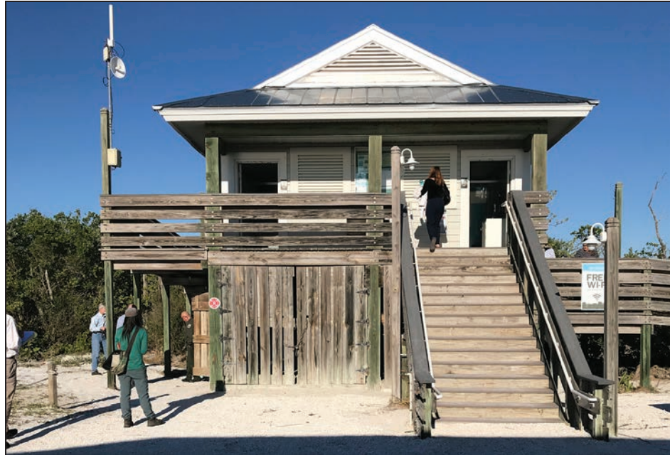
Figure 3-34: Elevated restrooms with ground-level enclosure. Lovers Key State Park restroom (Site 2; Lee County) enclosure sustained shallow flooding but no damage during Hurricane Irma.
