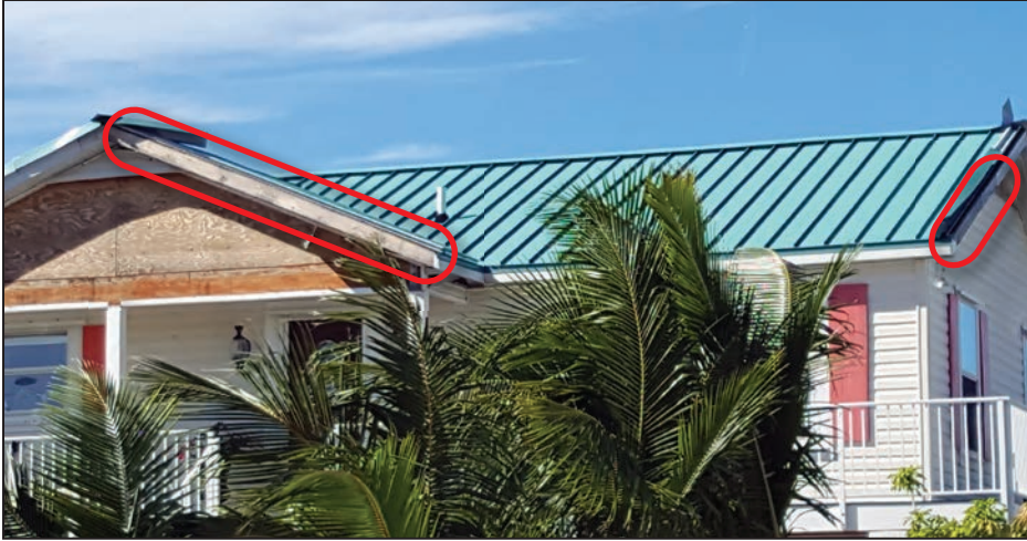
Figure 4-15: House with separated metal roof trim and missing fascia cover (red ovals) along gable end. (EWS = 113 mph; EDWS = 180 mph) (Sugarloaf Key)
