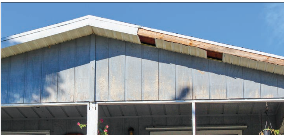
Figure 4-23: House with metal soffit loss below missing fascia cover (EWS = 114 mph; EDWS = 180 mph) (Big Pine Key)
