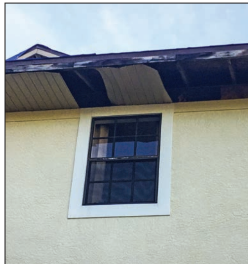
Missing metal soffit panels are shown below damaged fascia; located on the other side of the corner shown in left image.
