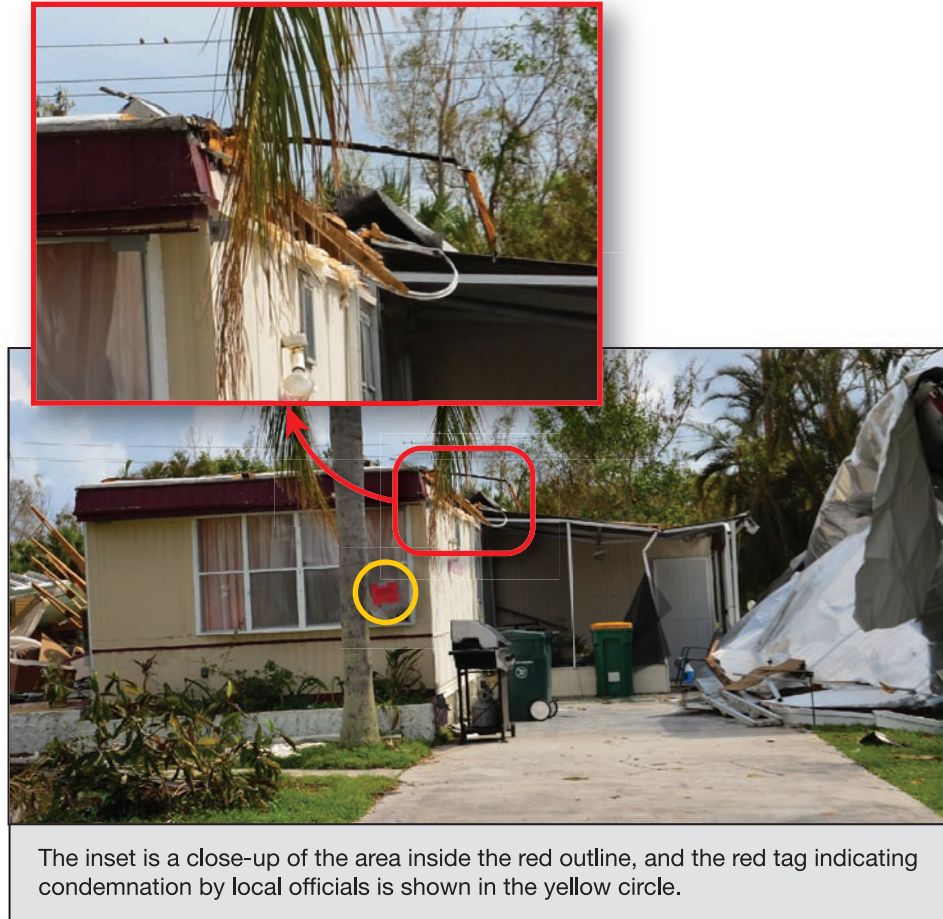
Figure 4-46: MH unit where carport detached from the unit, opening the building envelope across the top of a wall (EWS = 105 mph; EDWS = 166 mph) (Collier County)
