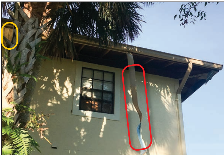
Dangling fascia cover (red outline) is shown adjacent to missing metal soffit panels near the corner of a Naples apartment building (yellow outline indicates intact soffit panels).
