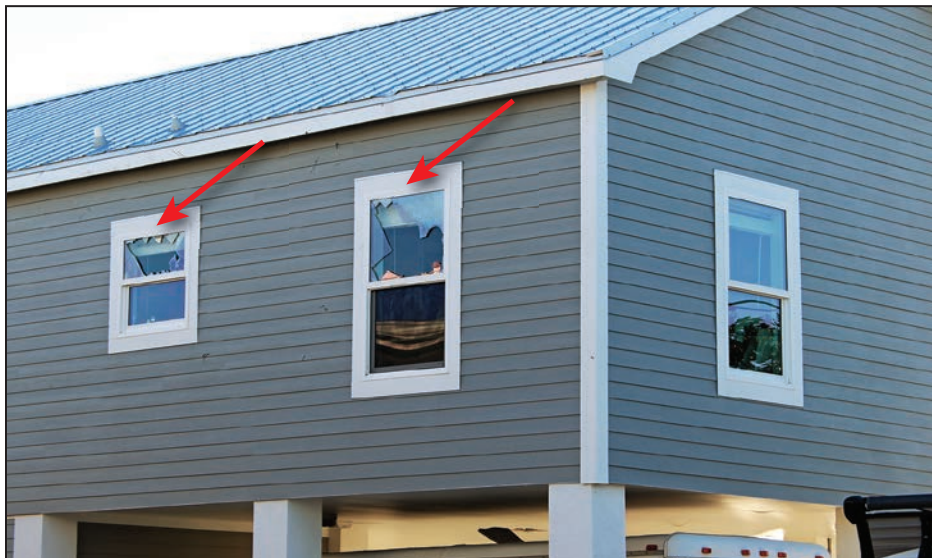
Figure 4-32: Residence with two windows where the outer panes were broken (see red arrows) but the inner panes stayed intact (EWS = 113 mph; EDWS = 180 mph) (Ramrod Key)
