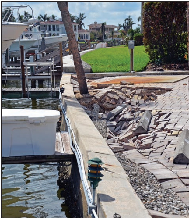
Figure 3-28: Bulkhead toe failure (insufficient embedment) (Naples, FL)
