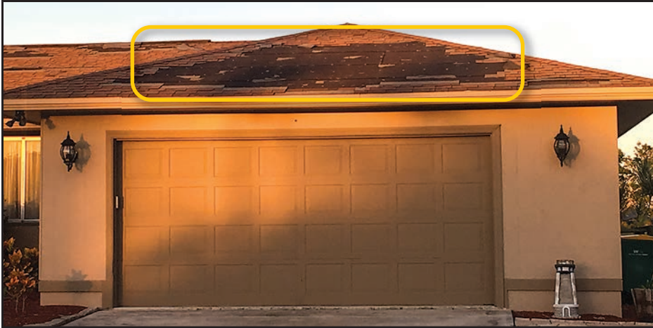
Figure 4-12: House with shingle loss near main ridge and between roof hips (yellow oval) (EWS = 109 mph; EDWS = 170 mph) (Marco Island)
