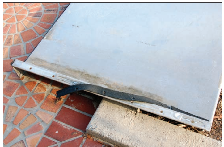
Figure 3: Torn gasket on metal flood panel after panel was removed. Gasket must be replaced before the next deployment.
