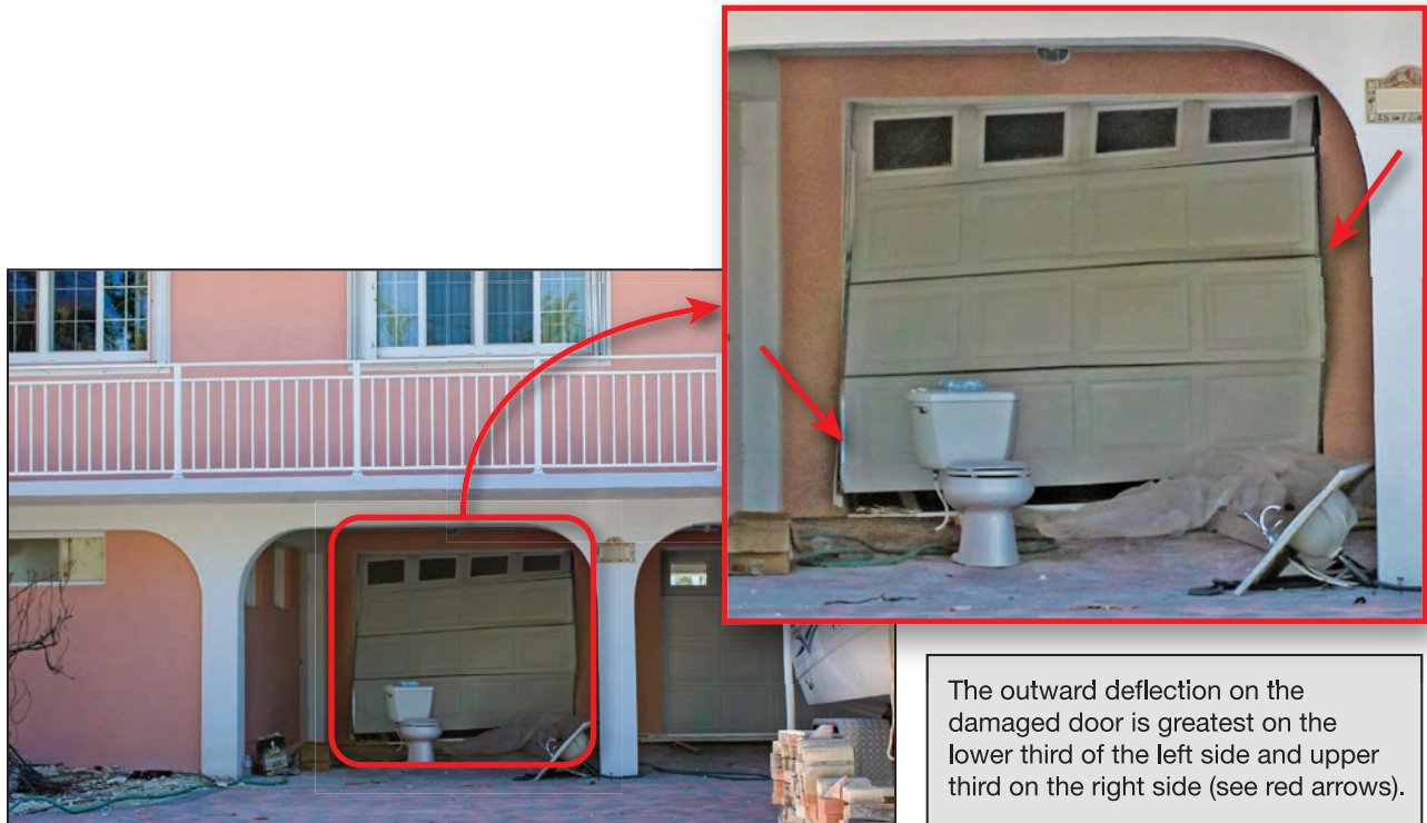
Figure 4-38: Damaged overhead garage door on a house (EWS = 111 mph; EDWS = 180 mph) (Duck Key)
