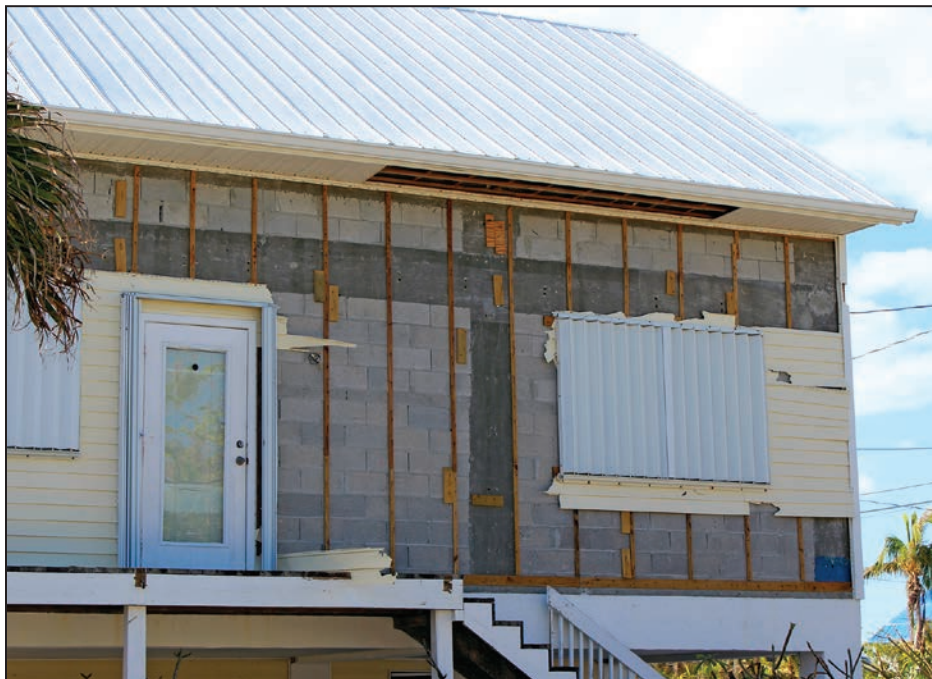
Figure 4-31: House with irregular fastener pattern and apparent lack of a proper starter strip (EWS = 114 mph; EDWS = 180 mph) (Little Torch Key)
