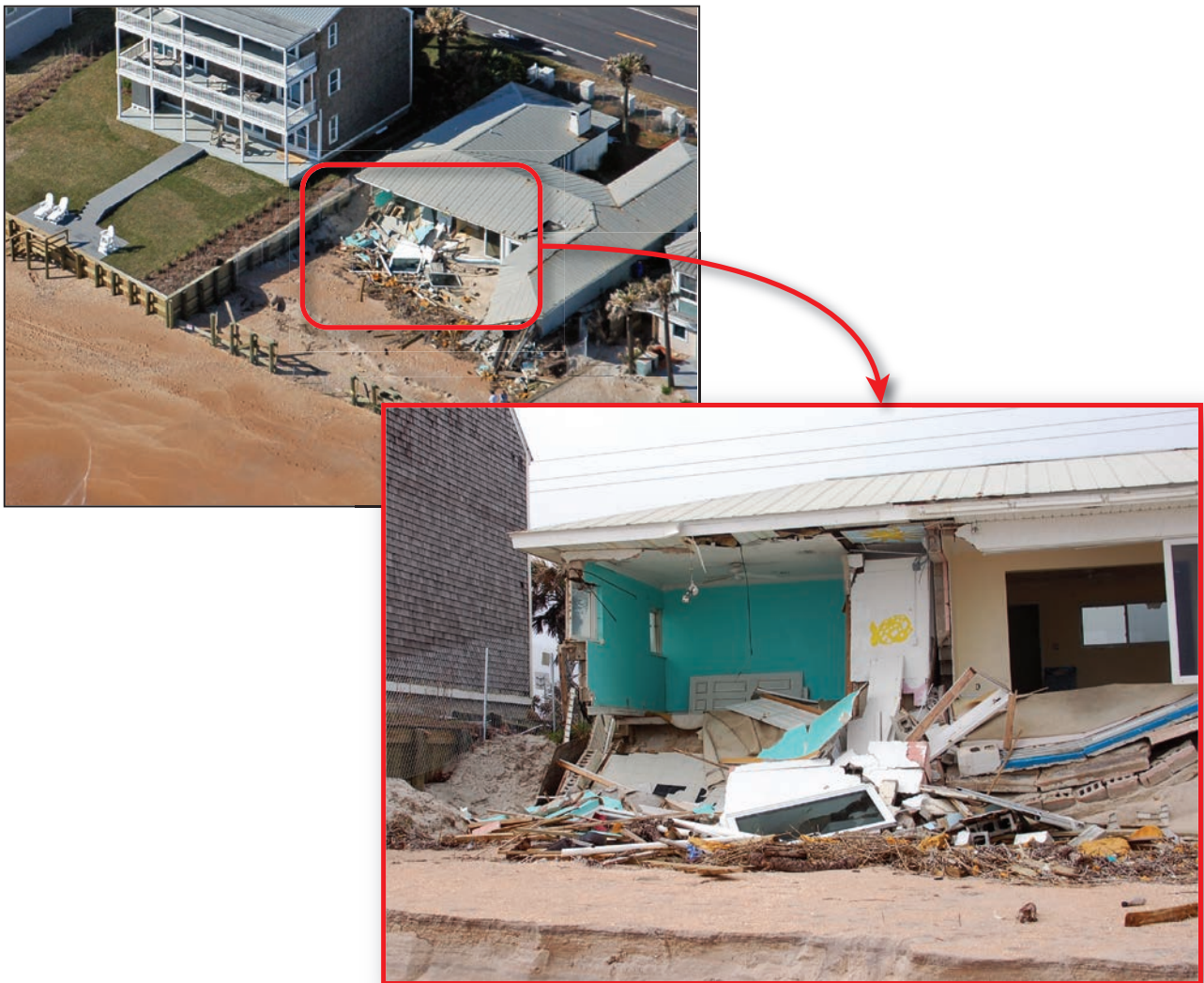
Figure 3-29: House on a shallow foundation that collapsed after it was undermined following failure of the bulkhead during Hurricane Irma (St. Johns County, FL)
