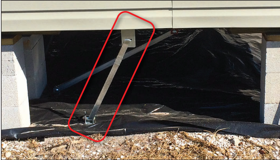
Figure 4-41: New MH unit installation with misaligned anchor strap installation (red outline) was otherwise anchored consistently with other post-Irma examples (EWS = 105 mph; EDWS = 164 mph) (Collier County)
