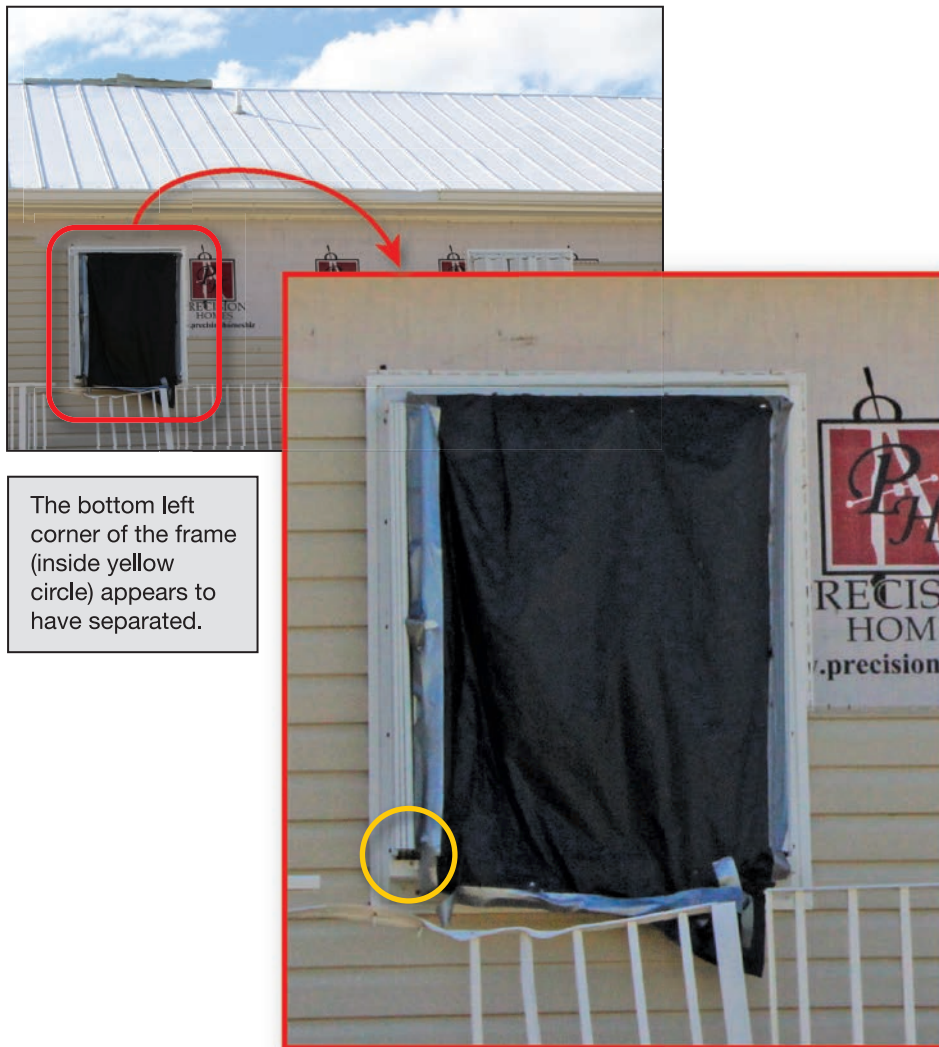
Figure 4-35: House with impact-resistant shutter system damaged by wind-borne debris; opening was covered at the time the MAT visited (EWS = 114 mph; EDWS = 180 mph) (Little Torch Key)
