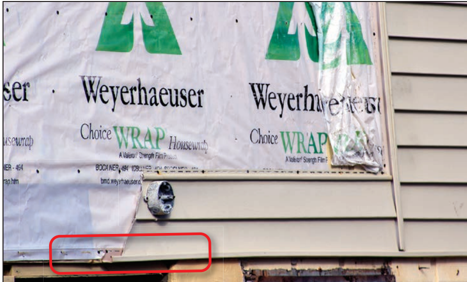
Figure 4-30: House that lacked a proper starter strip, as shown in the red outline (EWS = 114 mph; EDWS = 180 mph) (Little Torch Key)
