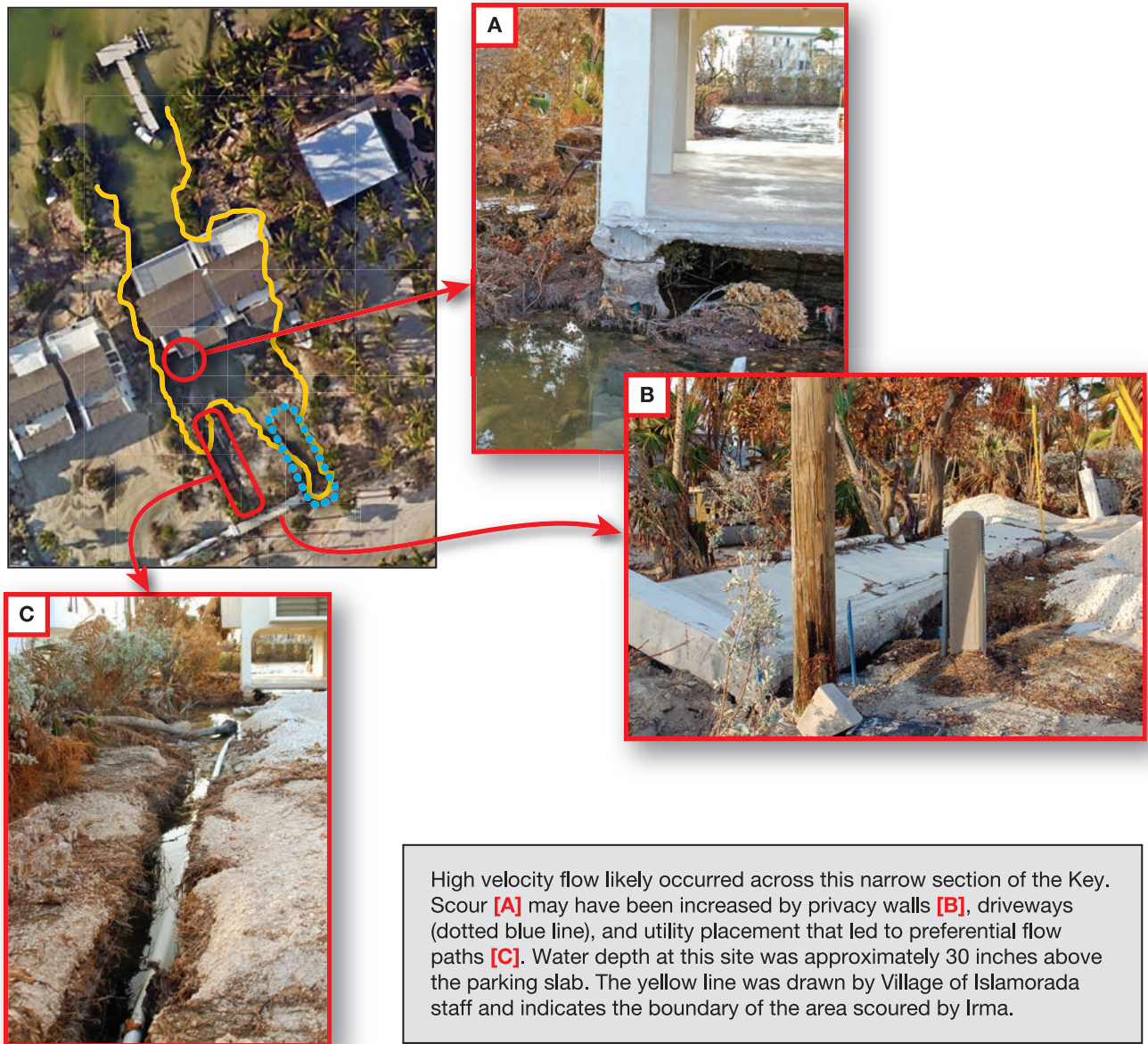
Figure 3-14: Scour near and around building foundation (Lower Matecumbe Key, FL)
