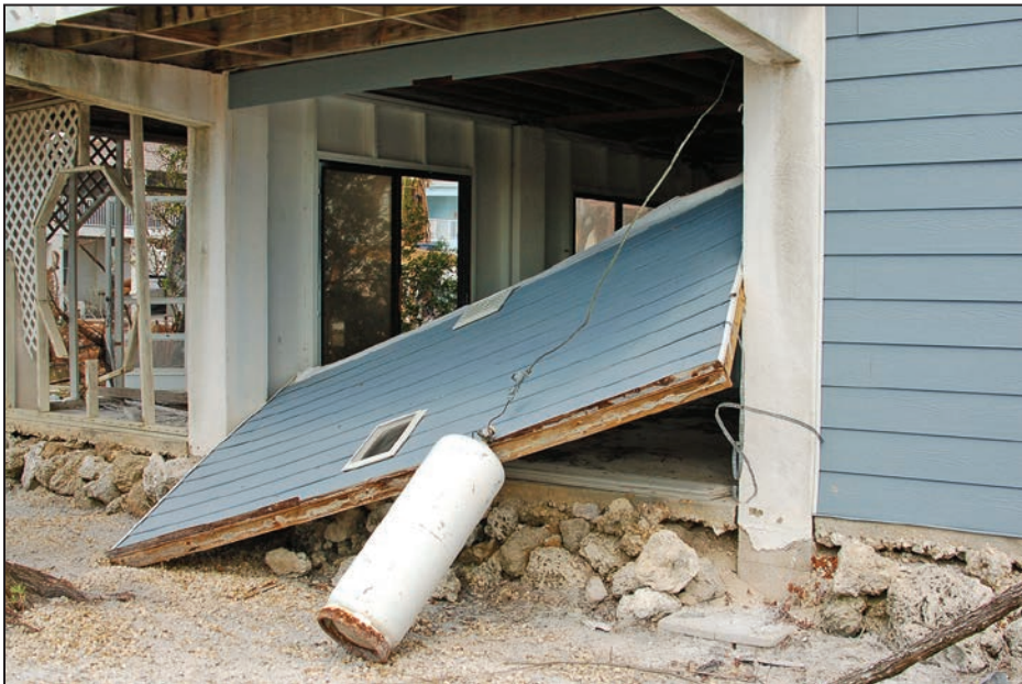
Figure 3-8: Example of partial failure of breakaway wall, with no associated damage to main structure observed (Cudjoe Key, FL)
