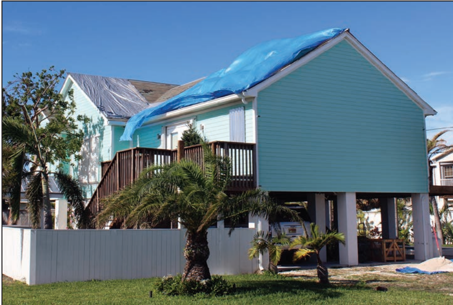
Figure 4-7: The MAT could not observe much of the asphalt roof damage on this house because it was covered by a tarp (EWS = 111 mph; EDWS = 180 mph) (Big Coppitt Key)
