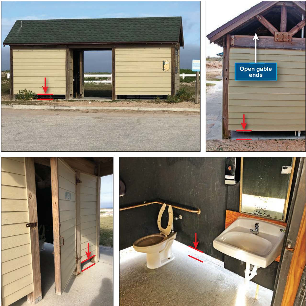
Exterior and interior photos of a restroom building at Surfside Park, St. Johns County. The wood frame outer walls do not extend to the floor slab (red arrows), and gable ends are open, allowing light and air to enter the restrooms. There is no electric service to the restrooms. The building likely sustained no flood damage during Irma.
