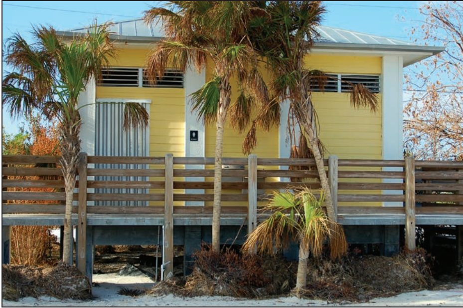
Figure 3-39: Elevated restrooms at Sombrero Beach Park without ground-level enclosure and that sustained no flood damage during Hurricane Irma (Site 7; Marathon)
