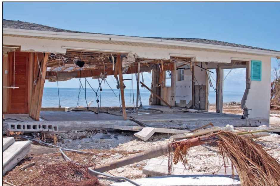
Figure 3-6: House constructed at grade where the masonry walls parallel to the shoreline were destroyed; this house was near the house shown in Figure 3-5 (Big Pine Key, FL)
