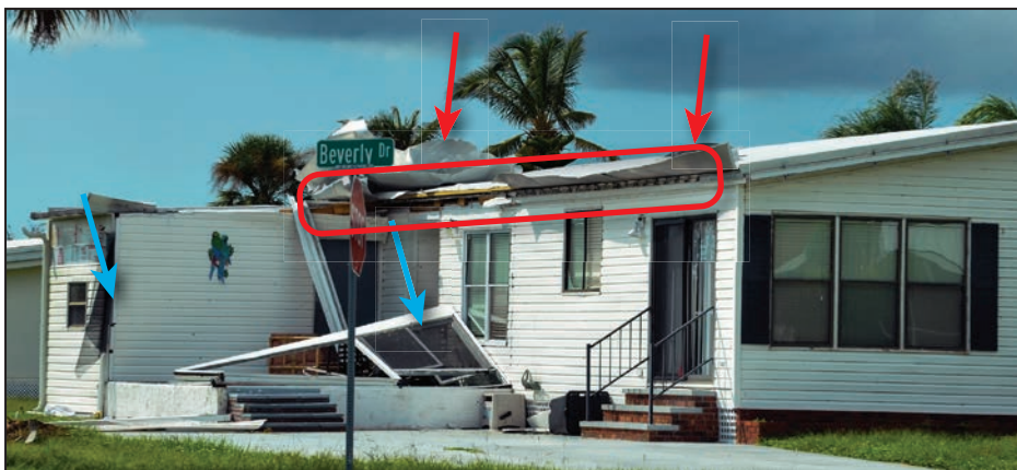
The screened porch (remnants shown with blue arrows) opened the top of an exterior wall (red outline) and peeled back the adjacent roof section (red arrows) when the porch was lost to high winds.
