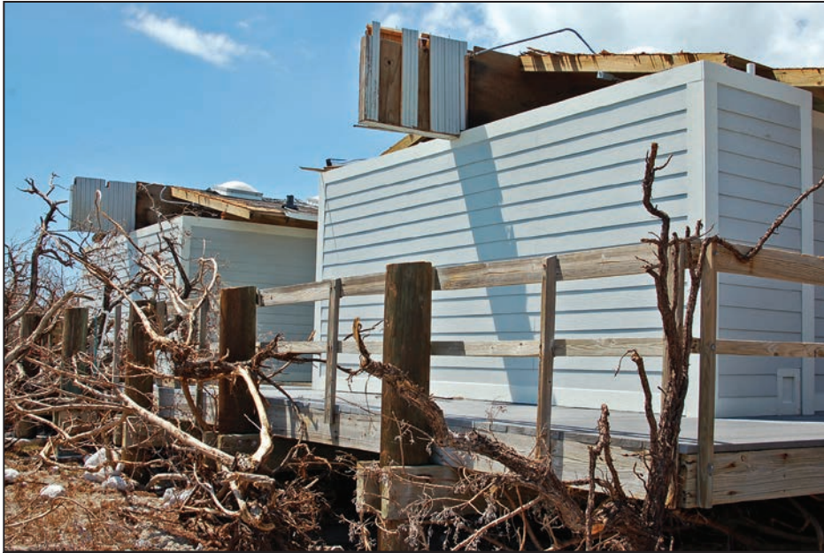
Figure 3-43: Elevated restroom at Bahia Honda State Park, Loggerhead (Site 13; Monroe County)
