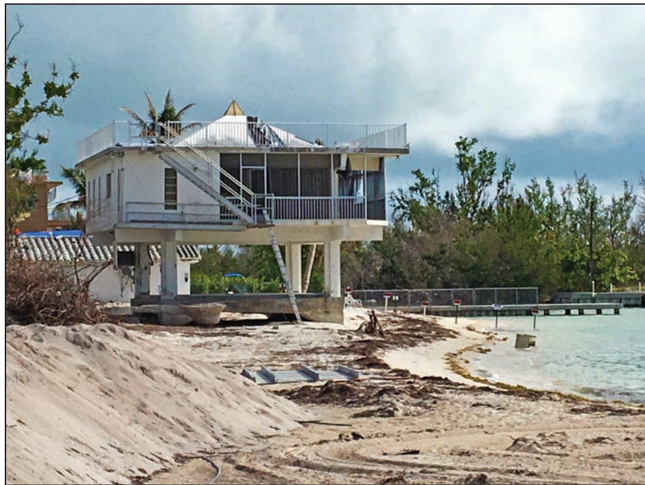
Figure 3-16: Erosion was likely due to wave attack around the foundation of this house on Sombrero Beach Road (Marathon, FL)
