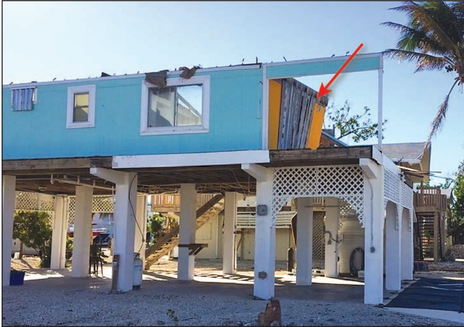
Figure 4-4: North end of east-facing wall where the roof was (EWS = 113 mph; EDWS = 180 mph) (Cudjoe Key)
