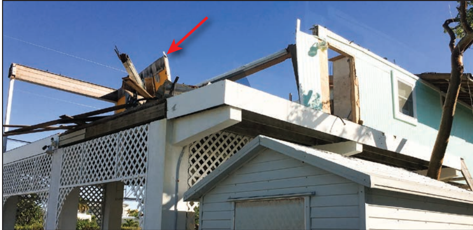
Figure 4-5: Remainder of the screened porch and exterior wall (EWS = 113 mph; EDWS = 180 mph) (Cudjoe Key)
