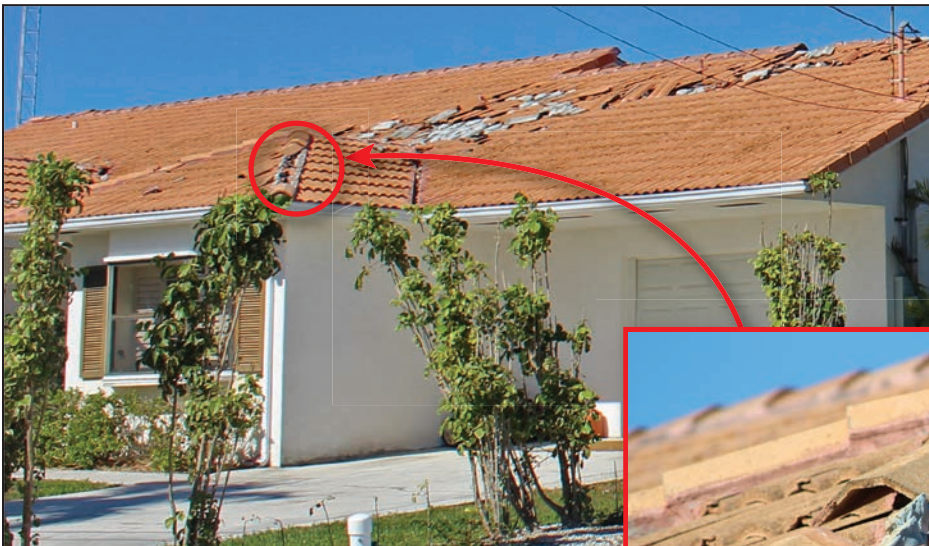
Figure 4-13: Roof tile failure (EWS = 113 mph; EDWS = 180 mph) (Cudjoe Key)
