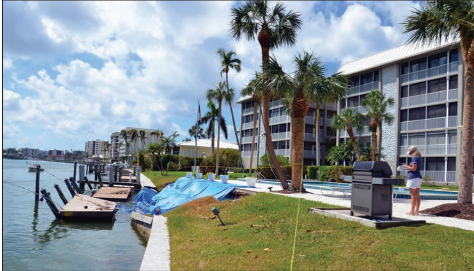
Figure 3-27: Failure of bulkhead (anchor system) (Naples, FL)
