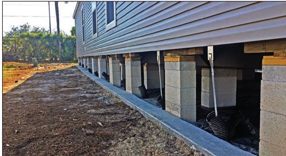
Figure 4-40: Consistent anchorage pattern observed on a new MH unit installation (EWS = 105 mph; EDWS = 164 mph) (Collier County)
