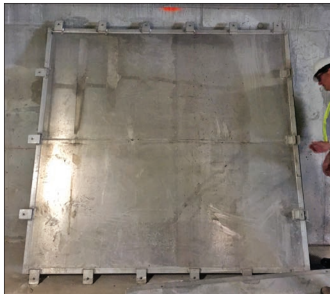
Figure 1: Large (6 feet high x 6 feet wide) metal flood panel requiring special equipment for installation
