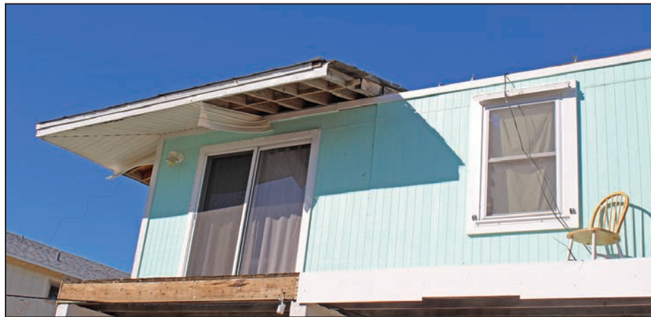
Figure 4-3: South end of east-facing wall; the south end of the roof remained in place (EWS = 113 mph; EDWS = 180 mph) (Cudjoe Key)
