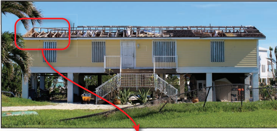
Figure 4-1: House with structural damage to roof system (EWS = 113 mph; EDWS = 180 mph) (Sugarloaf Key)
