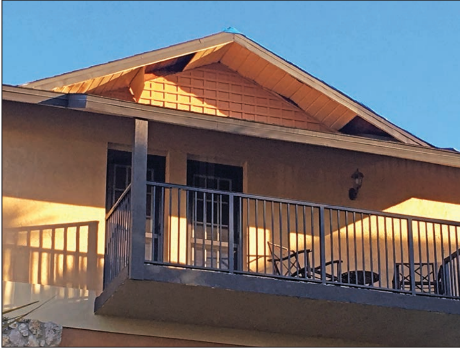
Figure 4-25: Metal soffit panel loss apartment gable end overhang (EWS = 104 mph; EDWS = 166 mph) (Naples)
