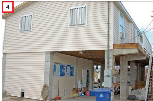
4 Minor enclosure damage to newer, elevated house situated away from the shoreline.
