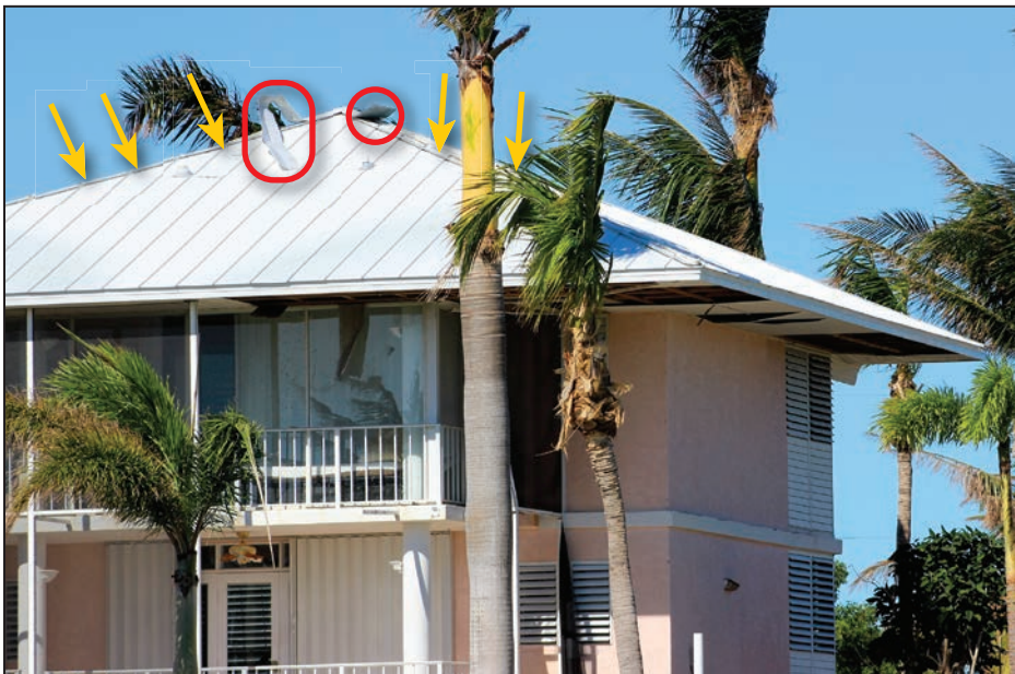
Figure 4-16: House with damaged metal roof system (EWS = 113 mph; EDWS = 180 mph) (Sugarloaf Key)
