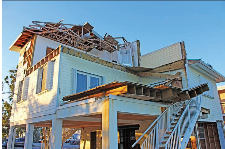
Figure 4-6: House with roof structure loss and collapse of the second floor exterior wall and adjacent deck (EWS = 113 mph; EDWS = 180 mph) (Ramrod Key)
