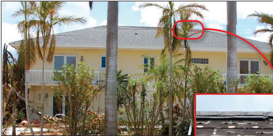
Figure 4-10: Residence that lost shingles near the ridge (EWS = 113 mph; EDWS = 180 mph) (Sugarloaf Key)
