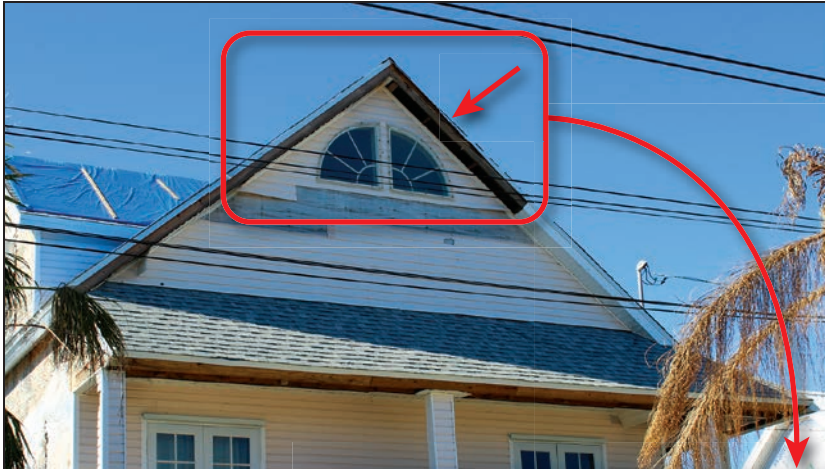
Figure 4-18: House that lost its soffit along the right side of the front-facing gable (EWS = 114 mph; EDWS = 180 mph) (Little Torch Key)
