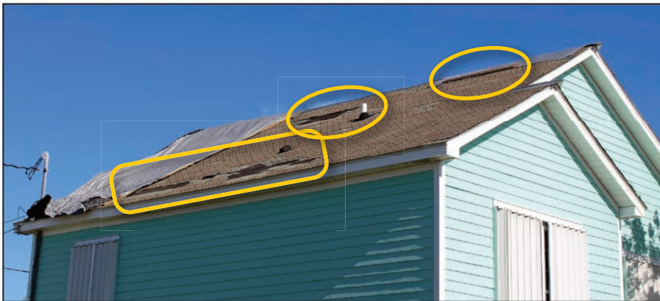
Figure 4-8: Asphalt shingle loss shown inside yellow ovals for house shown in Figure 4-7 (EWS = 111 mph; EDWS = 180 mph) (Big Coppitt Key)
