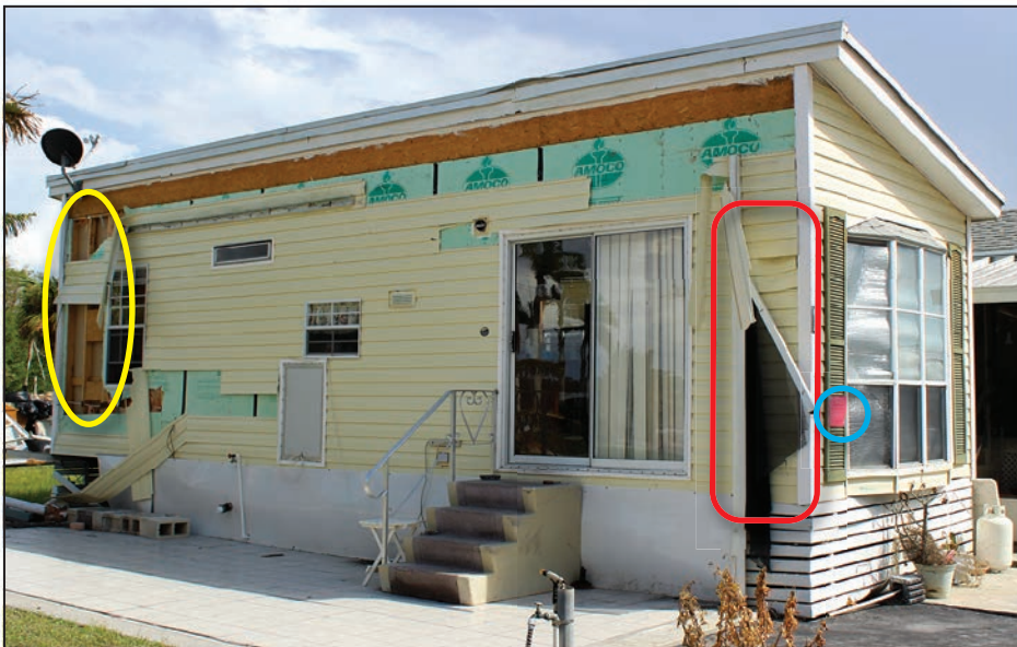
A remnant of the porch is shown in the red outline, and the red tag indicating condemnation by local officials is shown in the blue circle. The yellow oval shows missing sheathing and insulation characteristic of interior walls.
