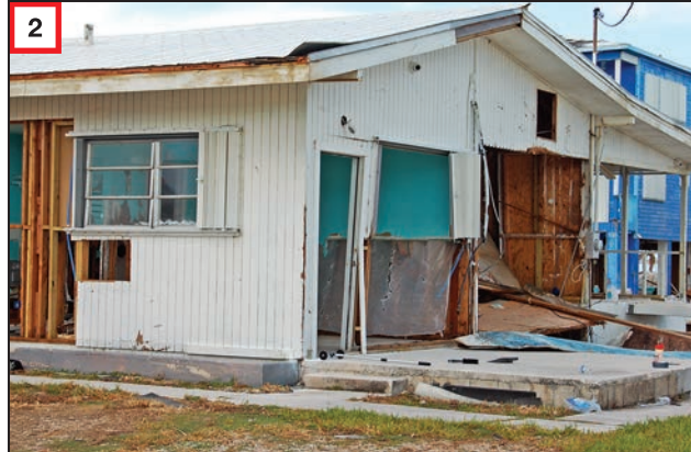
2 Inundation, water velocity, and debris damage to buildings situated farther from the shoreline.
