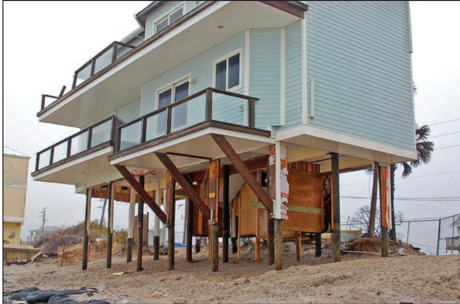
Figure 3-18: Undermined house on deep piles that survived erosion (Vilano Beach, FL)
