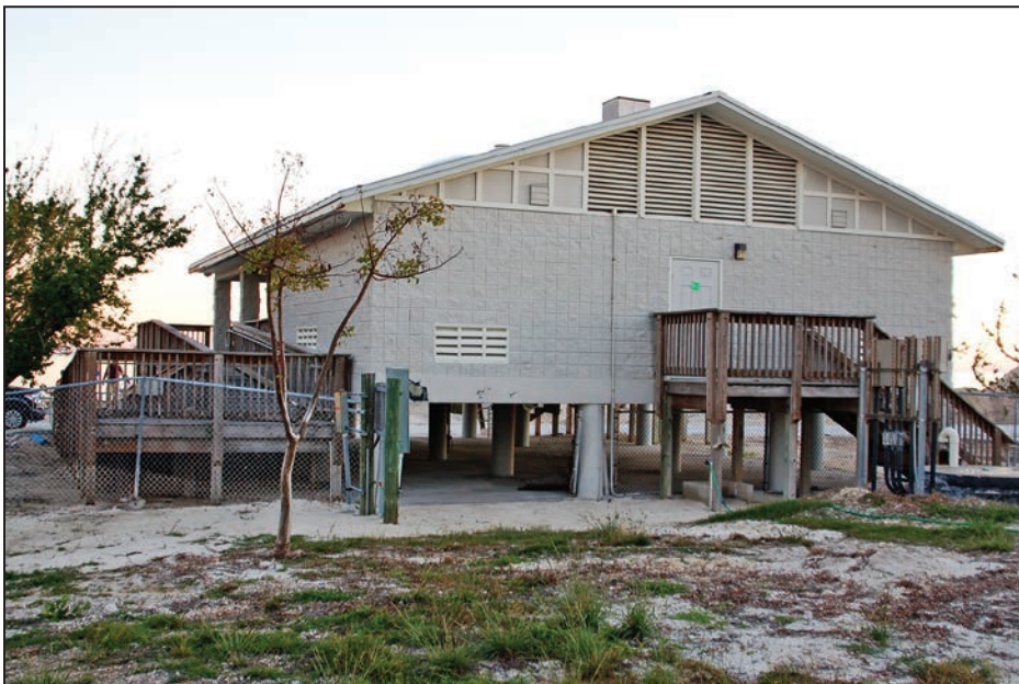
Figure 3-40: Elevated Long Key State Park restroom without ground-level enclosure and that sustained no flood damage during Hurricane Irma (Site 9; Monroe County)
