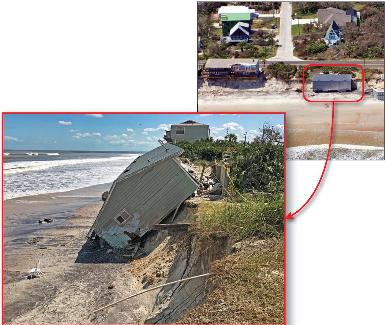
Figure 3-20: Collapsed house on shallow foundation that was undermined by erosion induced by Hurricane Irma (Vilano Beach, FL)
