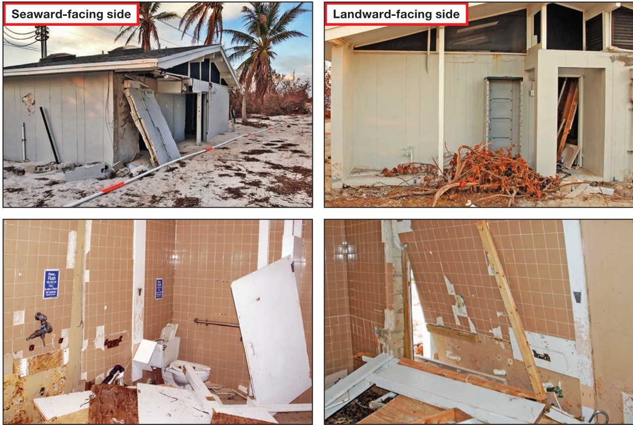
The bottom photos show damage to fixtures, partitions, and walls that was likely caused by waves and high-velocity flow. The restroom was demolished between the pre-MAT and MAT visits.
