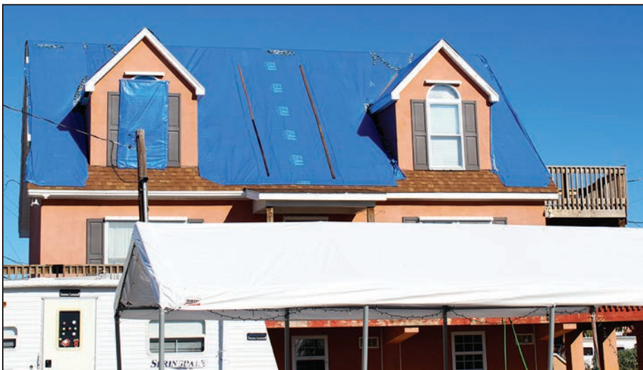
Figure 4-9: House with asphalt shingle loss as evidenced by tarp (EWS = 120 mph; EDWS = 180 mph) (Marathon)
