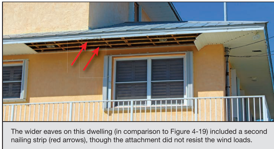
Figure 4-20: Dwelling with similar soffit panel attachment and loss as shown in Figure 4-19 (EWS = 113 mph; EDWS = 180 mph) (Sugarloaf Key)
