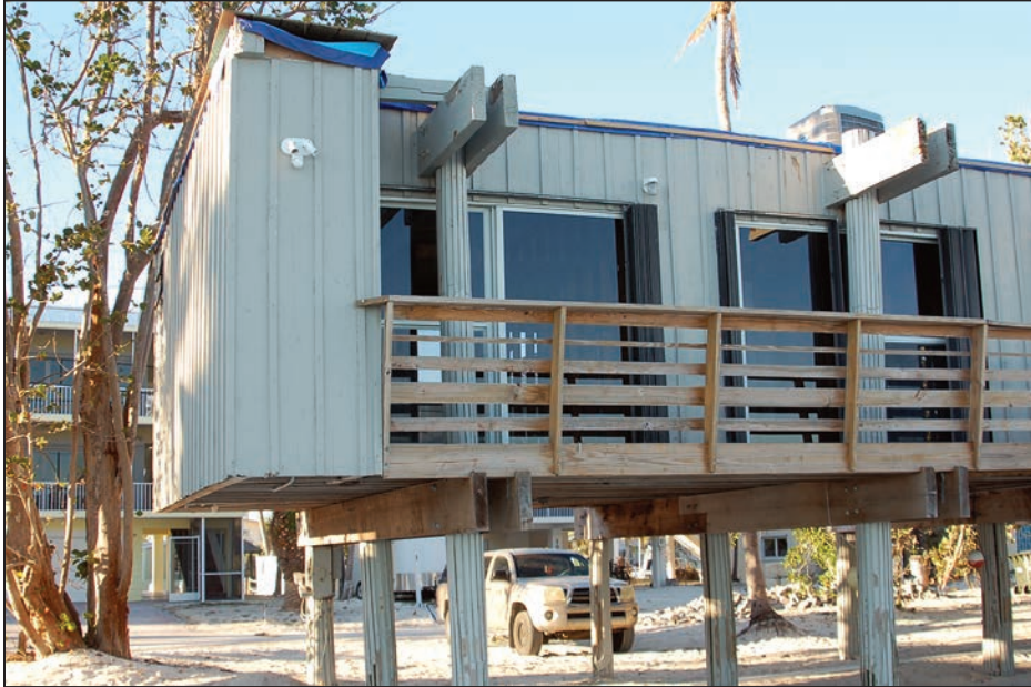
Figure 3-7: Example of a breakaway wall that was reported by a local code official to have performed as intended (Lower Matecumbe Key, FL)
