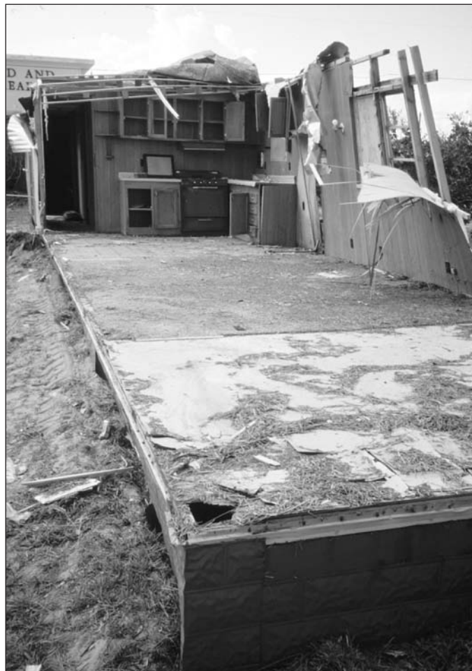
Figure 5-8. Failure of a modular home due to high winds. The home lifted off of its foundation (concrete slab) when the connections failed.
